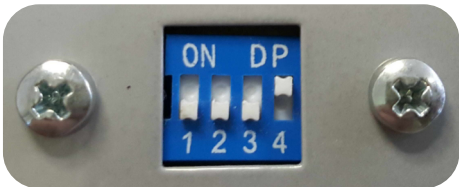
SWITCH (12-13) ON THE POLE
